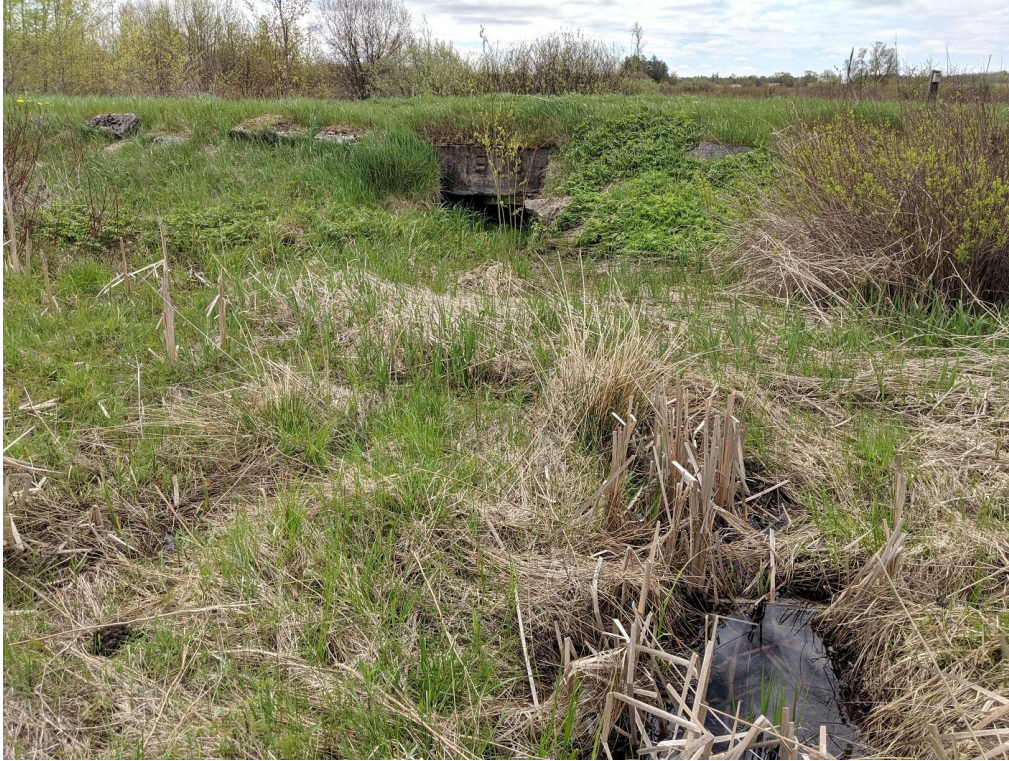
Photograph 3: West box culvert beneath the rail corridor located south of the pond (May 24, 2019).
