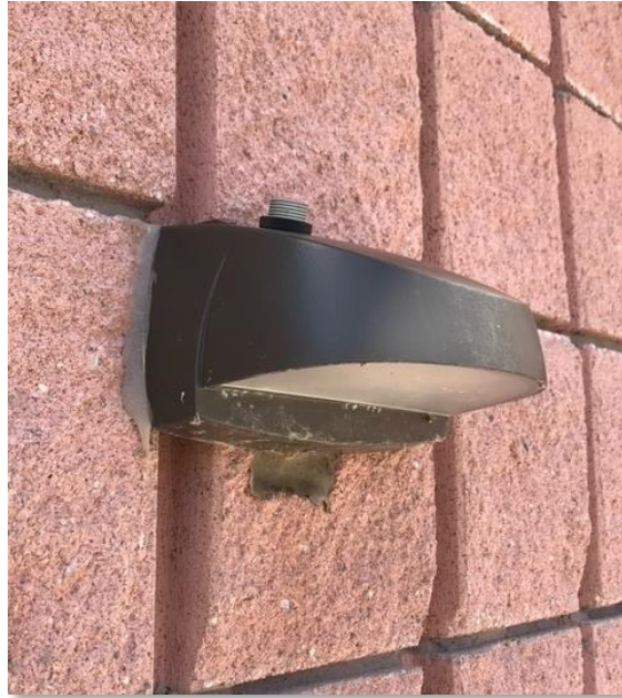
Figure 2.2 New LED Lighting Fixtures
