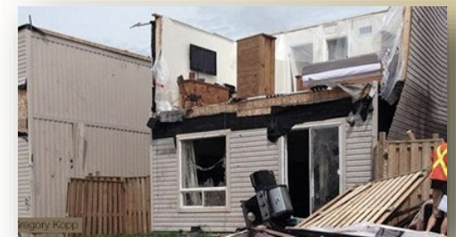
Damage from the Angus Ontario Tornado 2014
