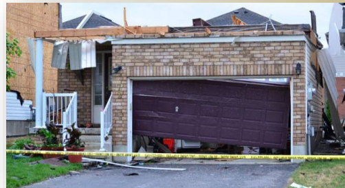
Damage from the Angus Ontario Tornado 2014
